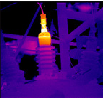
Figure 2. Heating on this oil-filled circuit breaker bushing is caused by high-resistance in the connection between the cap and the bushing rod.
