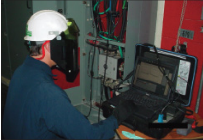
Figure 1: PPE requirements are taken into account per NFPA 70E
