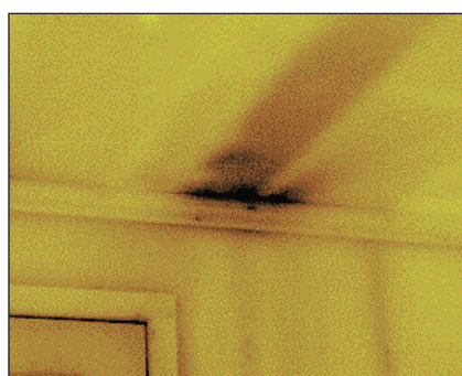
Figure 5: Batt insulation is susceptible to air infiltration. The fiberglass shown here does not stop airflow directly into the home or indirectly into the ceiling section.
