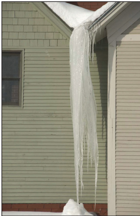
Figure 1: Icicles like this are a good indication of poorly performing insulation and/or ventilation.
