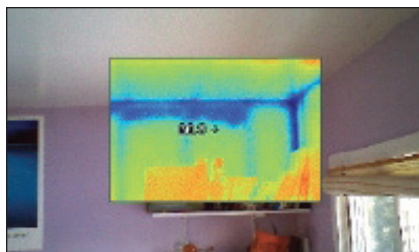
Figure 4: Properly installed cellulose is an excellent insulation. Unfortunately it is often poorly installed with missed areas and settling the most common quality problems.
