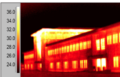
Image 11: During the commissioning of this building thermography revealed an extreme problem involving exfiltration through the soffit. Courtesy Phil McMullen.
