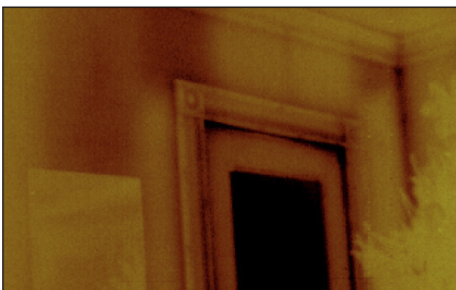
Image 4: Properly installed cellulose is an excellent insulation. Unfortunately, it is often poorly installed with missed areas and settling the most common quality problems.
