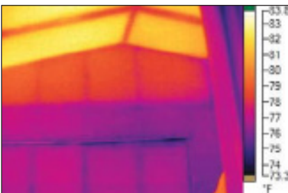
Image 7. The thermal pattern of apparent missing insulation between the roof joints is clearly seen at the top.
