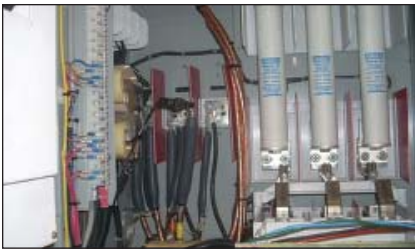
The guilty culprit: defective insulator
