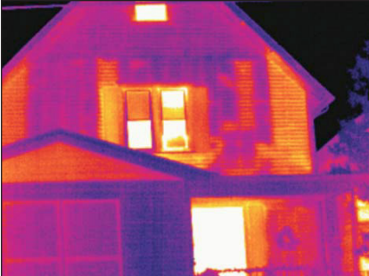
Image 2. The thermal image of this heated building during cold weather conditions clearly shows areas of apparent missing insulation on the second floor.
