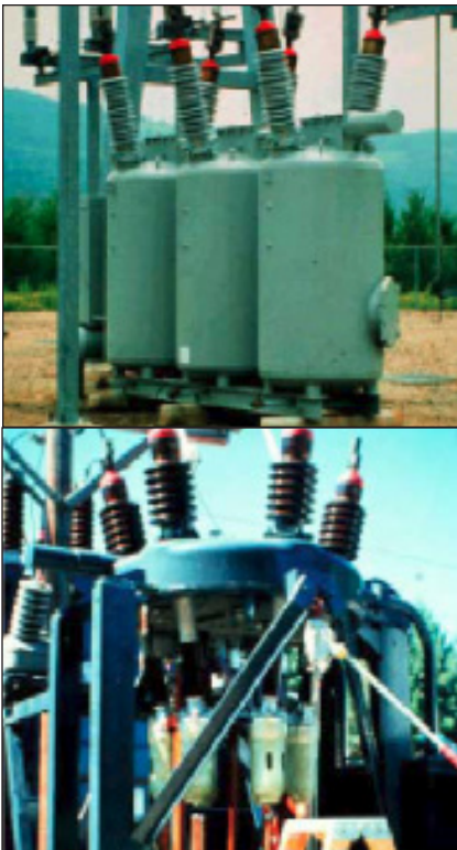
Figure 1. A set of 3-phase oil-filled circuit breakers (OCBs) seen from the outside (above) and another set (below) from the inside, with the oil drained, showing part of the bushing structure and contacts.
