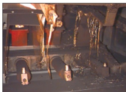
Figure 1d: Catastrophic (or Critical) Failure
