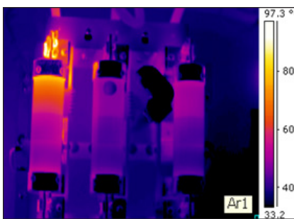
Figure 5b: Potential Failure
