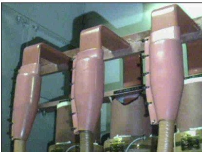
Figure 2. These connections provide power to a 15,000 HP critical motor. Failure of this connection could result in a $1,000,000 per day outage.
