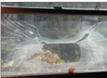
Imploded window with gaping oval hole in the inner glass.
