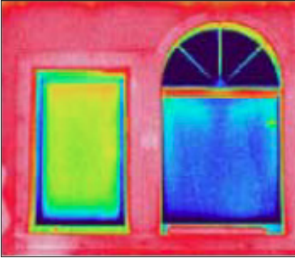
The relative thermal performance of three windows: single-glazed (top), double-glazed with nitrogen gas (right) and double glazed with argon-fill (left), is readily apparent in this thermogram taken from inside during the heating season.
