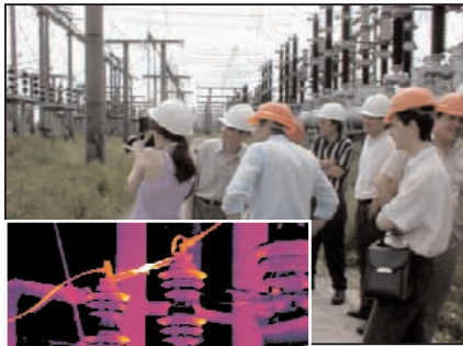
Inspecting the power station; problems found at switchyard. (insert)
